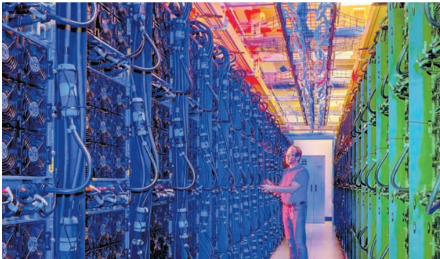
Microsoft's cloud server rows at its data center in Quincy, Wash., in an undated handout photo. As bigger companies slide onto the data-storage market, Box, Dropbox and Hightail are rethinking their core business models, focusing on specific industries or bolstering customer service.
